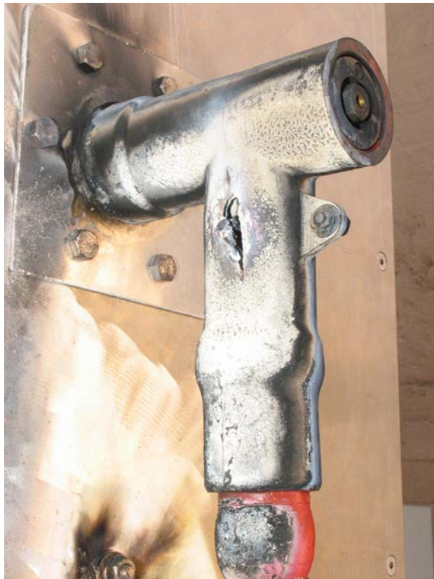
Figure 17: Test object No. 10 after the screen fault current initiation test at U_o = 12.7 kV (solidly earthed systems)
