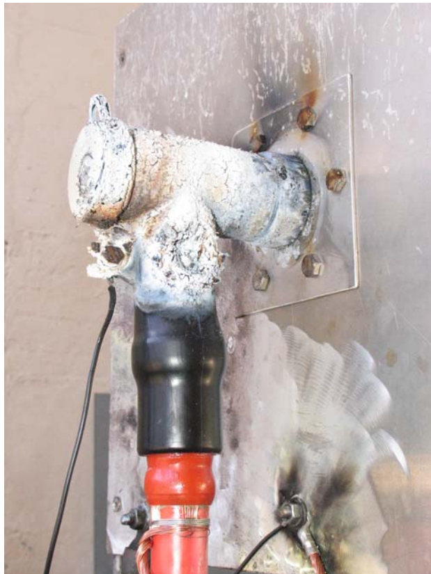
Figure 21: Test object No. 11 after the screen fault current initiation test at U_o = 12.7 kV (unearthed or impedance-earthed systems)
