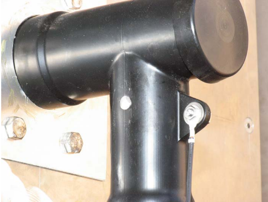
Figure 16: Test object No. 10 before the screen fault current initiation test (solidly earthed systems), point of arc initiation
