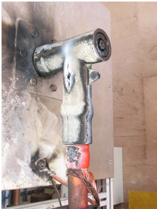
Figure 18: Test object No. 10a after the screen fault current initiation test at U_o = 6.35 kV (solidly earthed systems)
