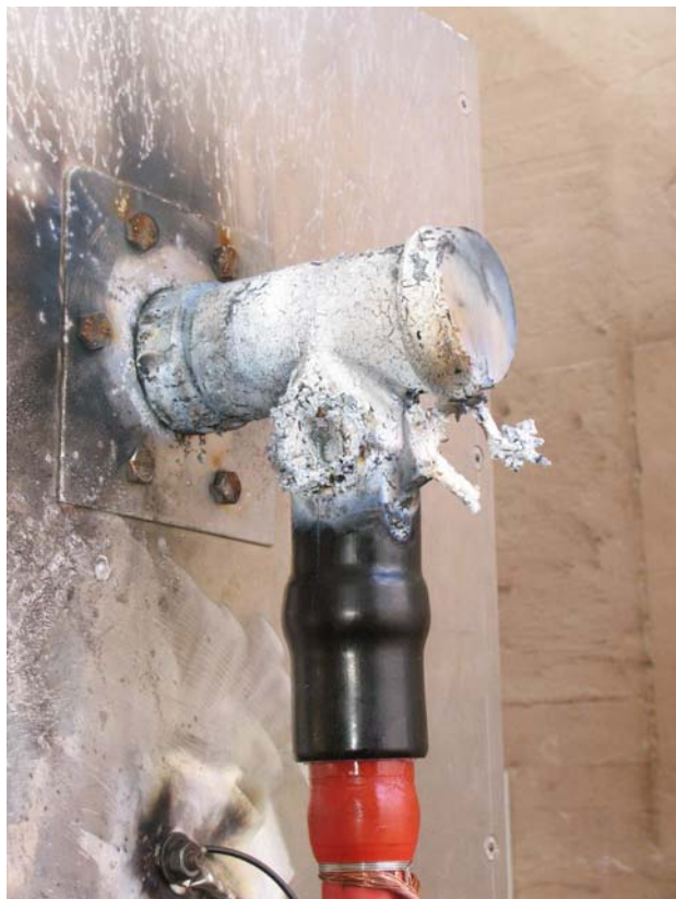
Figure 22: Test object No. 11a after the screen fault current initiation test at U_o = 6.35 kV
