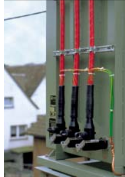
Screened Elbow Adaptors installed on outdoor SF 6 -transformer.
